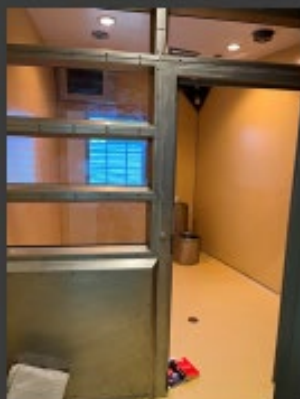
SASH Cell viewed from the airlock
