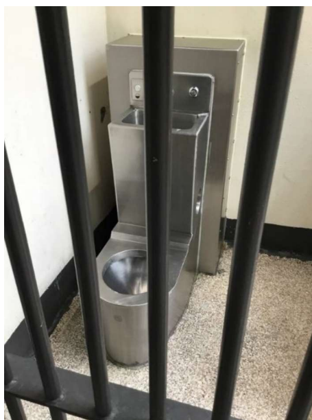
Launceston Reception Prison day yard toilet
